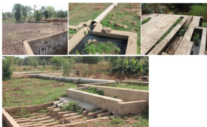
Figure 10: Waste Water Treatment System for Military Barracks in Tamale
