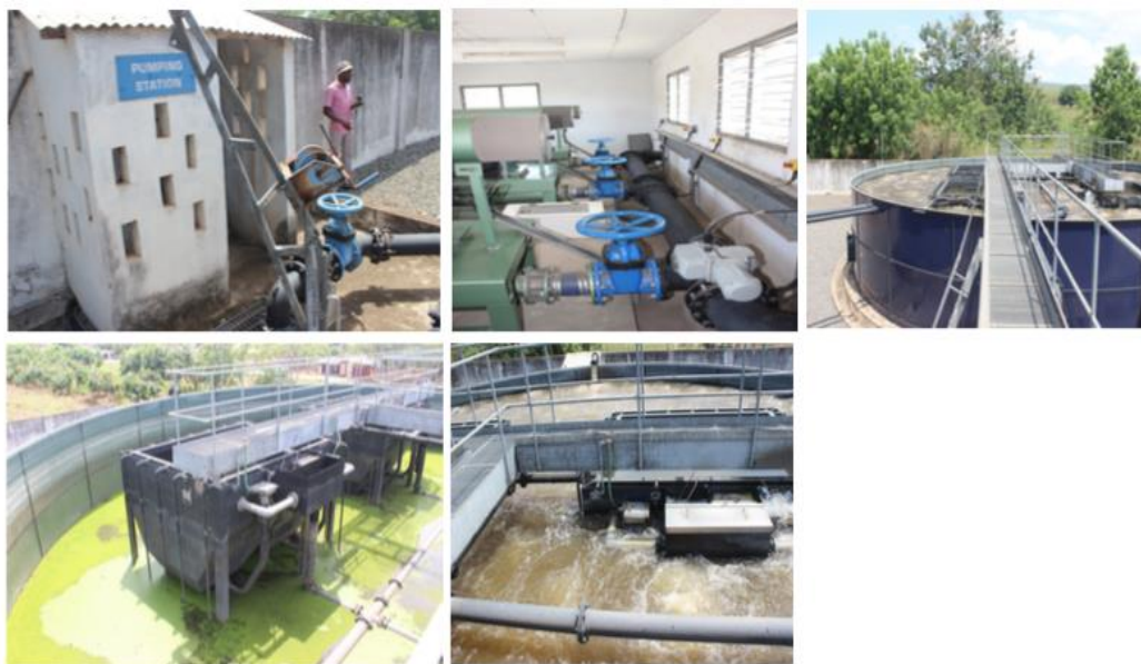
Figure 7 Components of the Wastewater Treatment Plant in Ho
