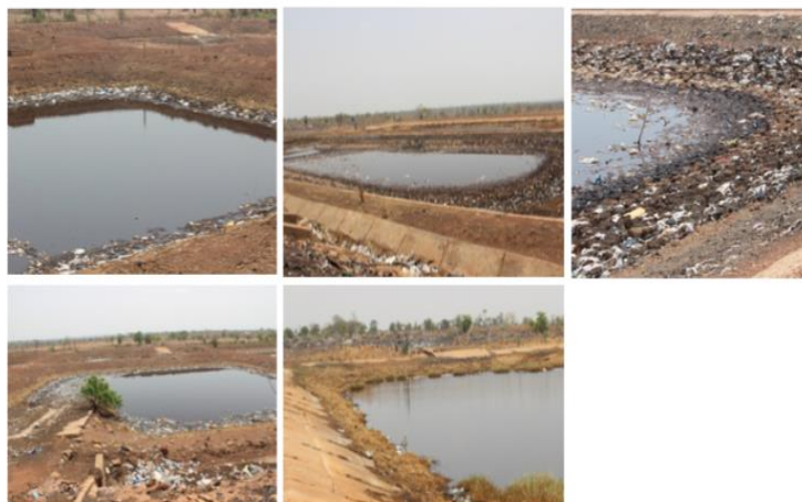
Figure 9: State of various components of Waste Stabilization Ponds
